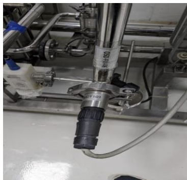
Fig.9 Feed Water Sampling Point
