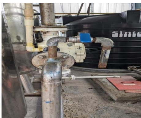
Fig. 8: Raw Water Sampling Point
