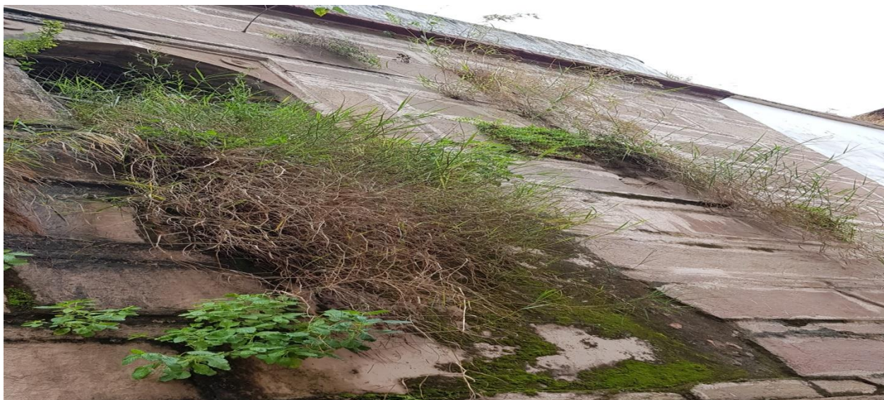
Fig.3: Walls of Akshay Vat of Allahabad Fort showing microbial induced deterioration
