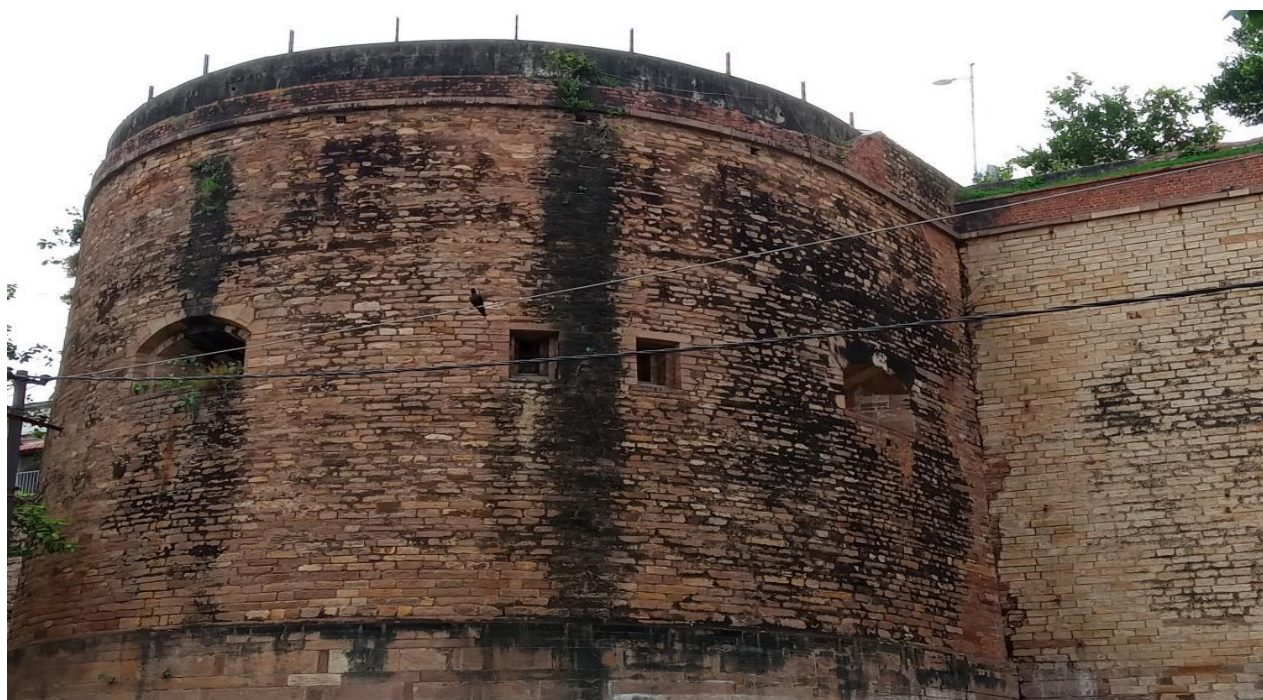
Fig.2: Walls of Allahabad Fort showing microbial induced deterioration
