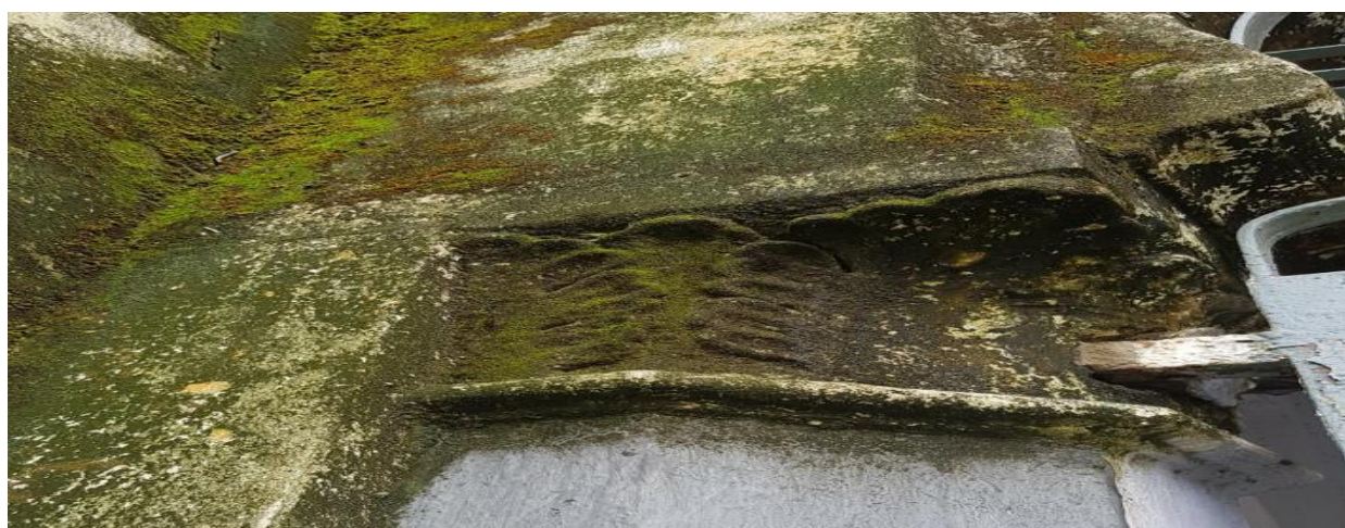
Fig.1, Wall showing Microbial biofouling, discoloration and staining (Senate Hall of University of Allahabad)
