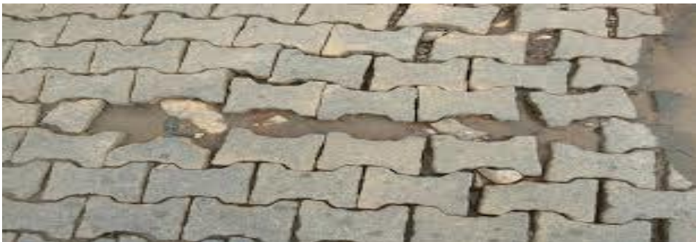
Figure .5 Settlement of bedding material due to this uneven surface appear.
