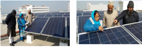
Fig 4. 150 kW SPV System
